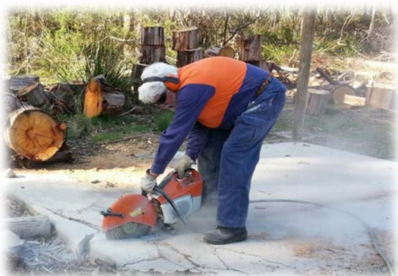
Jeff G cutting off the old shelter slab, making way for Indoor Range drainage.
